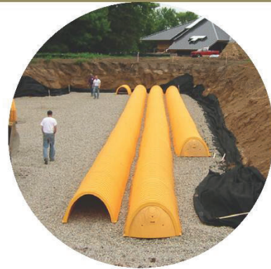
Below-Ground Recharge Systems
