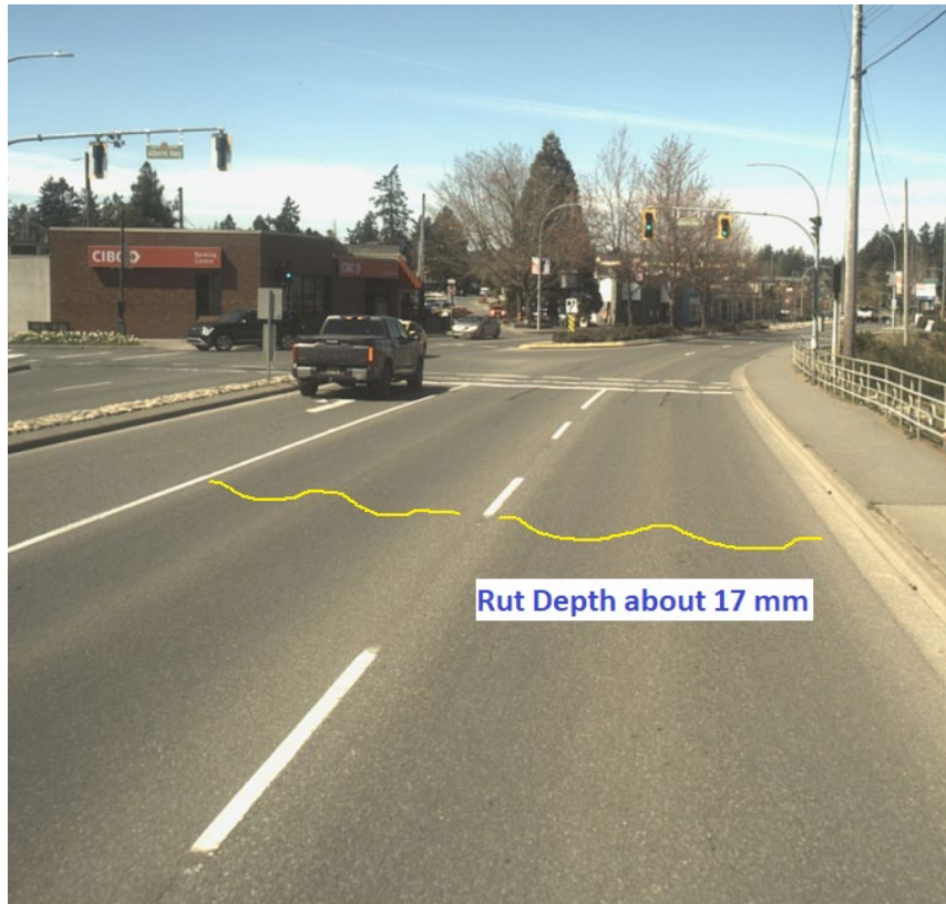
Figure 8: Moderate Severity Rut- Segment located on Island Highway West
