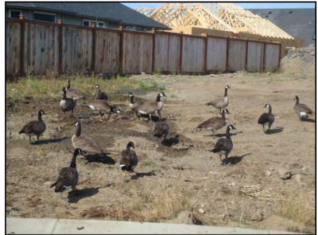
Canada Geese enjoying a leaking hose at a building site in Parkville, August 17, 2009
