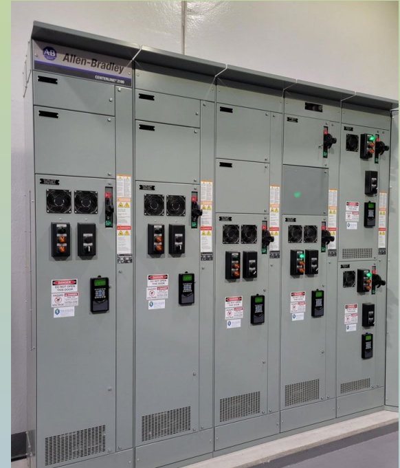
Allen Bradley Motor Control Centre
